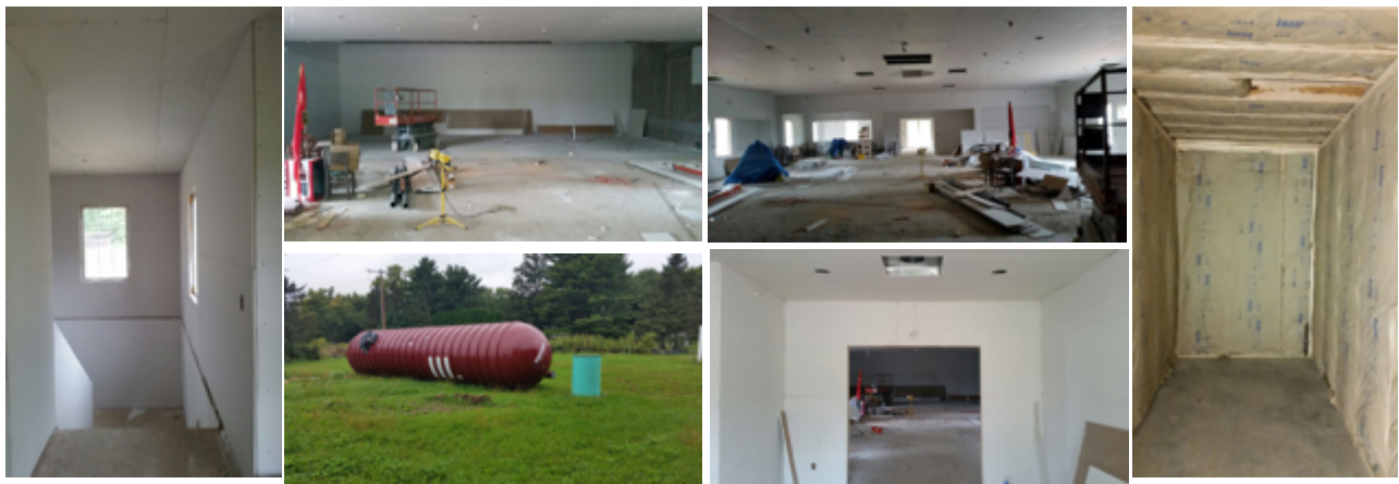
The Temple and Community Center Building: Interior and Exterior Works in Progress
